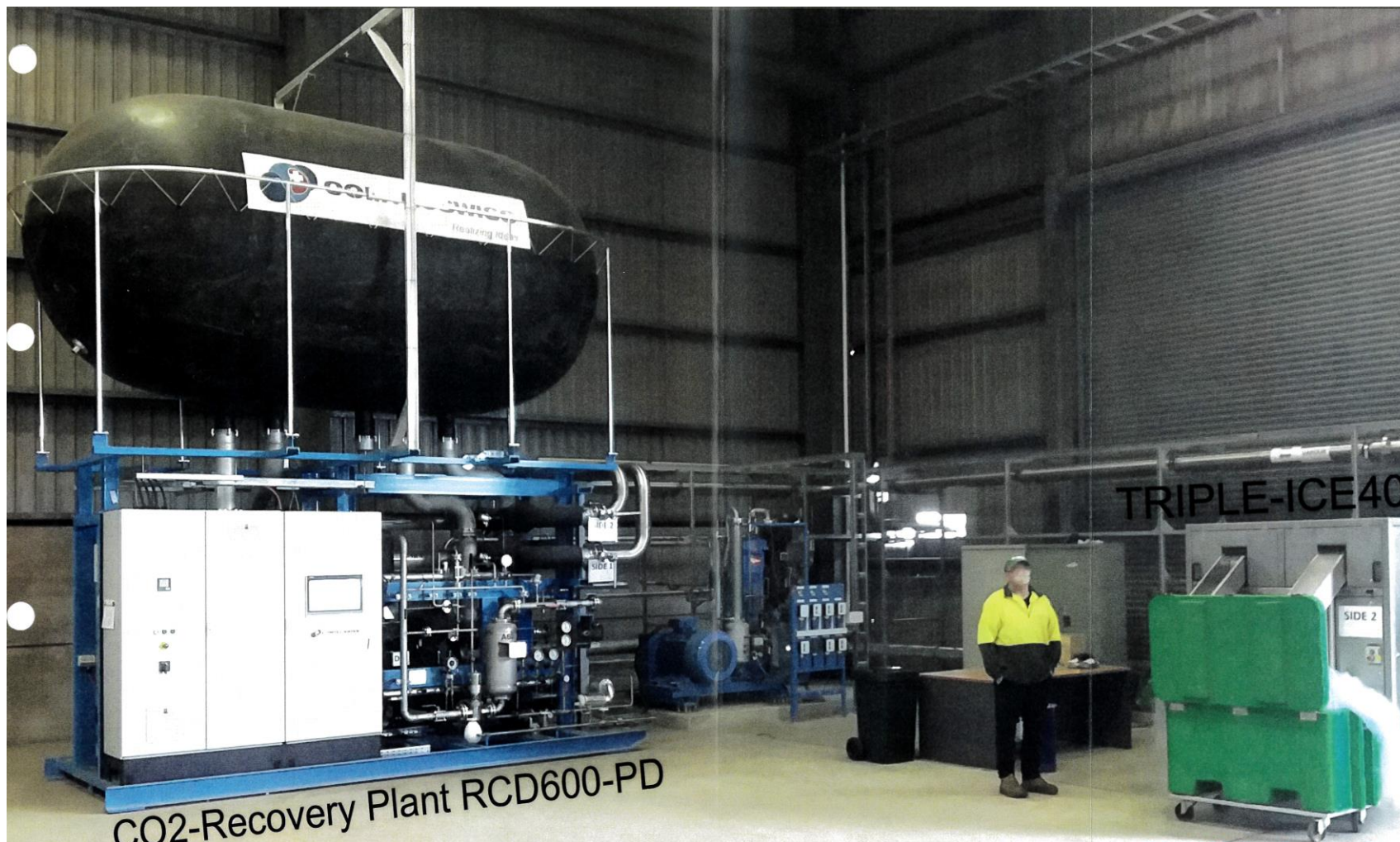
CO2-Recovery Plant RCD600-PD Comtecswiss 2023
